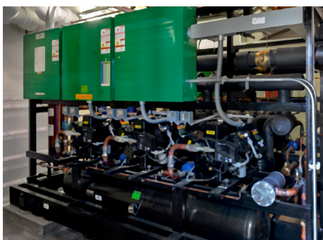
Synthetic Refrigerant Chiller
