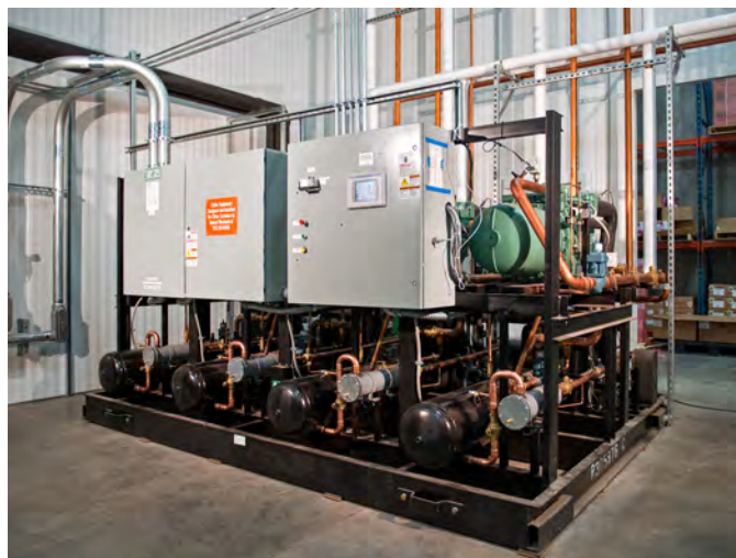
Industrial Chiller System
