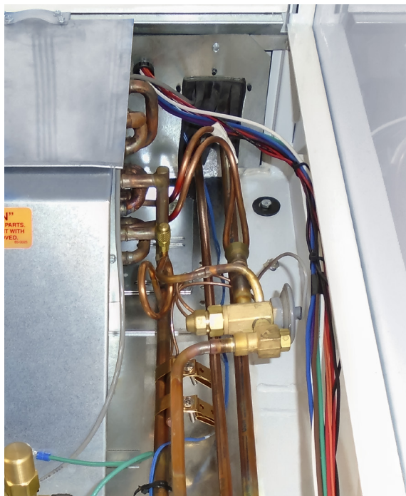
FIGURE 30: Expansion Valve Next to Evaporator Coil
