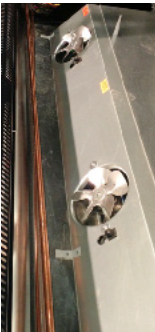
FIGURE 29: Fans and Case-to-Case Piping
