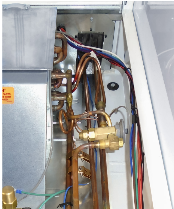
FIGURE 30: Expansion Valve Next to Evaporator Coil
