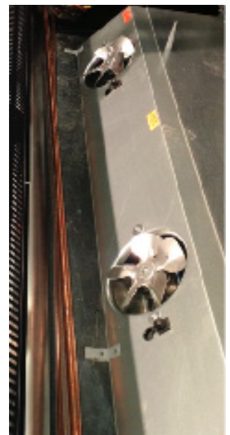
FIGURE 48: Fans and Case-to-Case Piping
