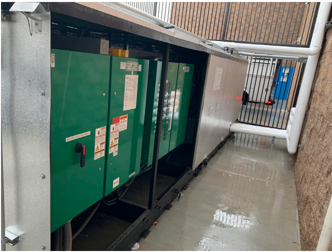
Power Distribution Panel
