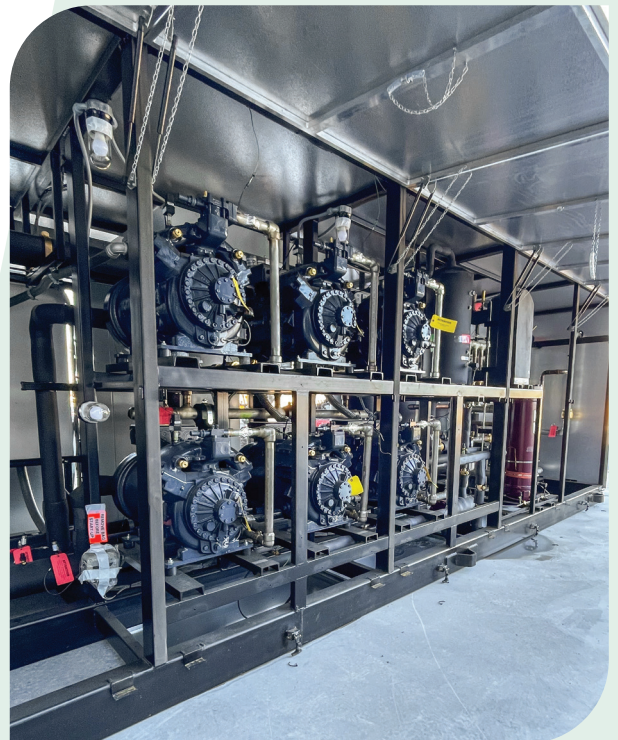
Outdoor Parallel Rack - Arkansas
