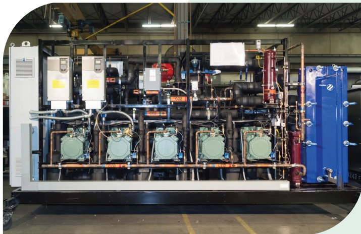
Transcritical CO 2 Chiller Rack - San Francisco, CA.
