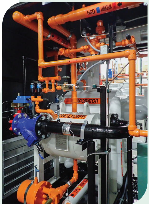
Water-Cooled Ammonia Chiller - Louisville, KY.
