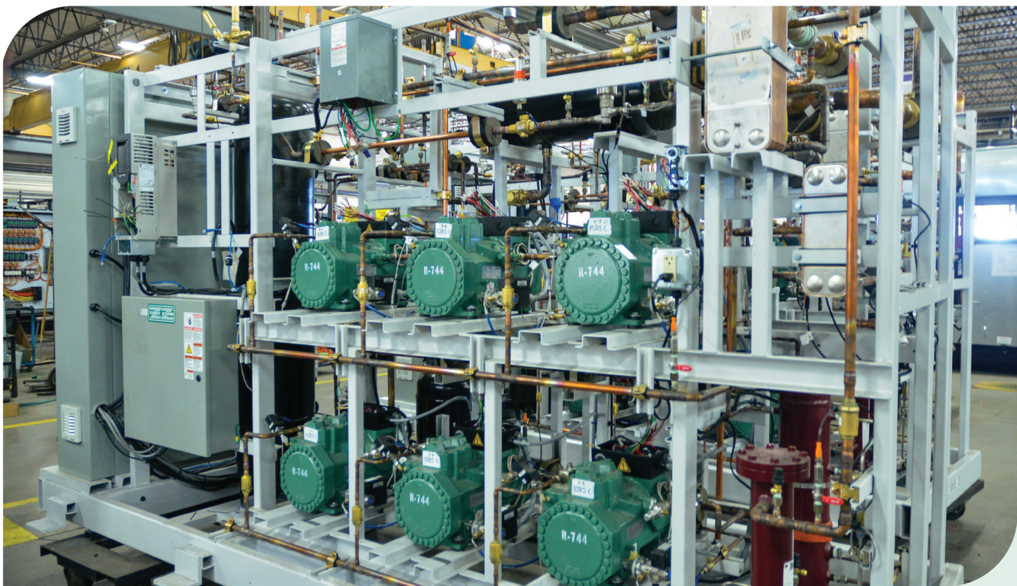
Transcritical CO 2 Chiller Rack - Oceanside, CA.
